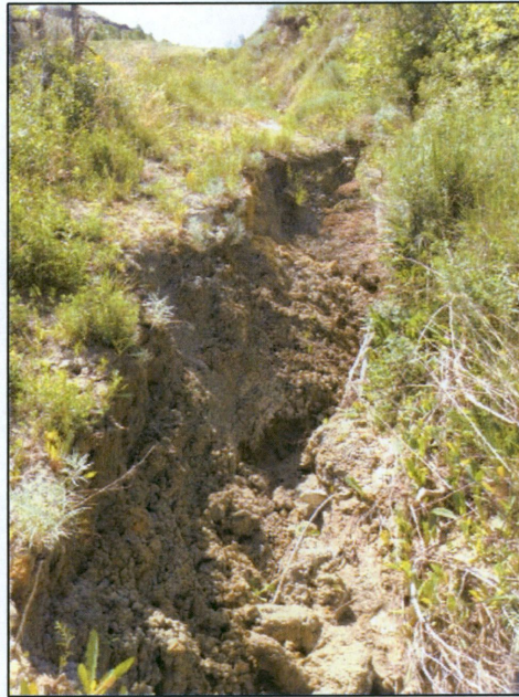
Photograph 11. Incising channel along western margin of fill area. View to southeast.
